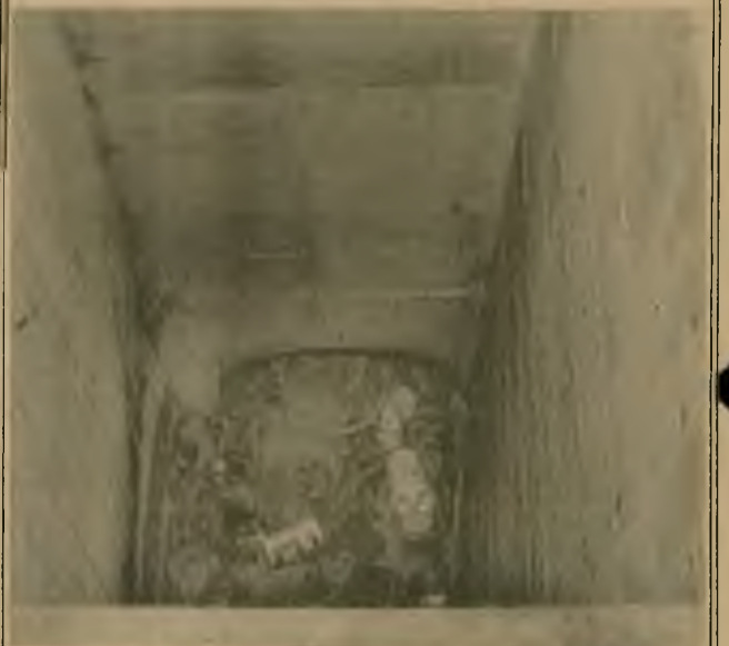
Pictured above is "The Pit," an eight-foot-deep cement hole next to Ashton Hall. What purpose it serves we do not know. What we do know is that it is a dangerous hazard for the many small children who play in the area. A child could easily fall in this uncovered menace and be hurt or trapped. Plant services should rectify the situation immediately.
